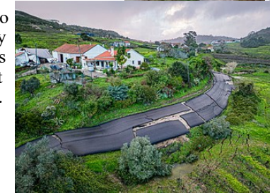
A badly damaged road following the recent storm.
